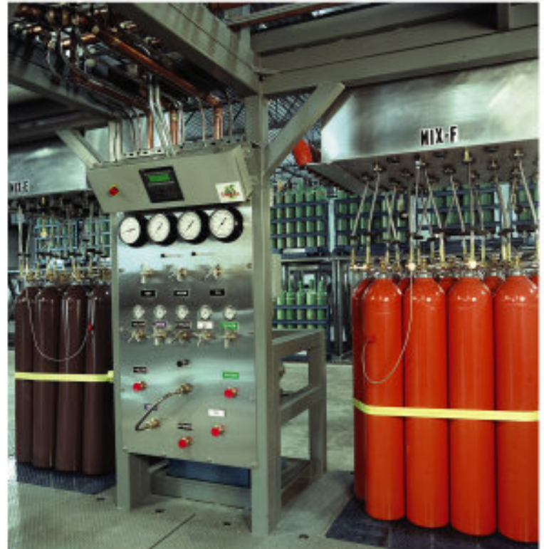
Inert Gas Filling Station
