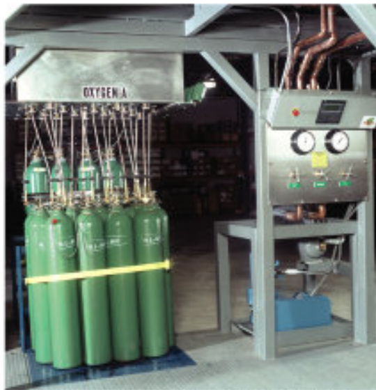
Oxygen Gas Filling Station
