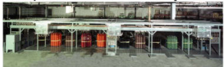
Gas Filling Island with 3 Filling Stations
